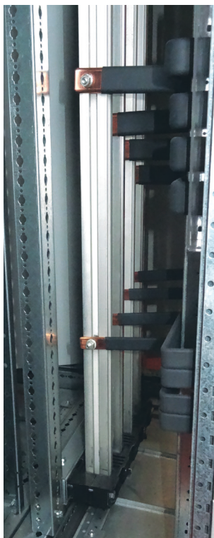
Busbar installed in cable sleeve.
